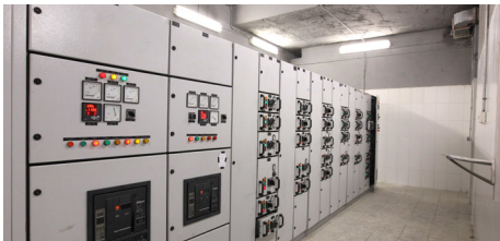
Electrical & Electronic Cabinets
